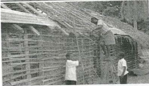
A teacher from Miembe Saba Primary School in Yombo ward, Bagamoyo district, Coast region, Ayoub Mruthu constructs a house worth Sh80, 000 after he was asked to shift from his previous house that was supposed to be occupied by a secondary school teacher. The house, which was half way finished, was demolished after the issue was published in this paper on March 22, 2006.
